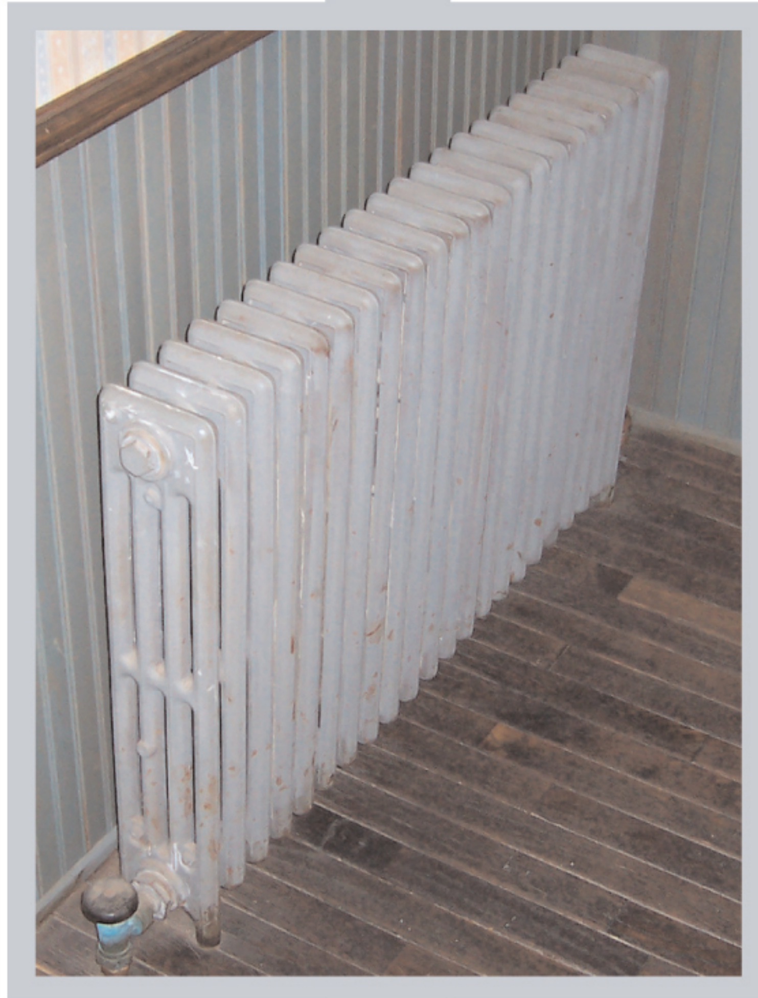
Old style heavy, bulky cast-iron radiators
